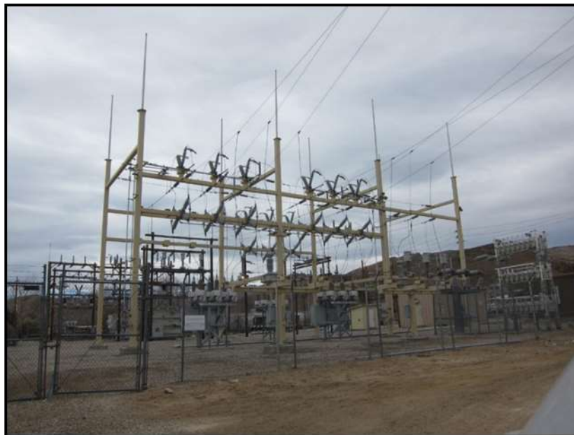
Figure 5 Silver Peak Electrical Substation
